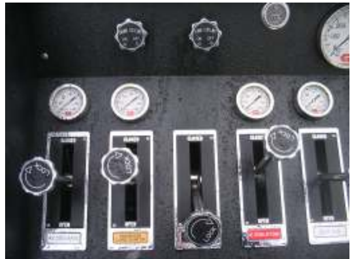
Top Control Fire Pump Panel
