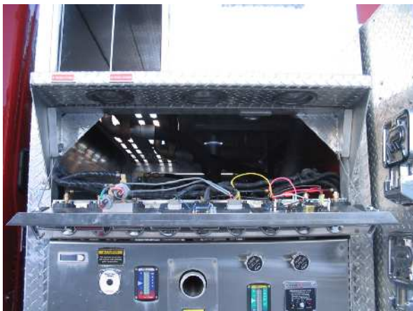
RIGHT SIDE FIRE PUMP PANEL
